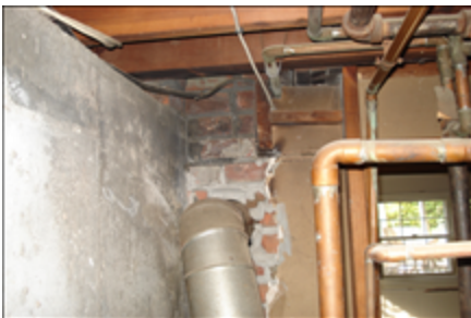
Unsealed Flue Pipe Entry
