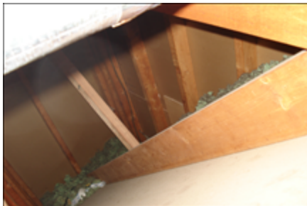
Uninsulated Attic Gap
