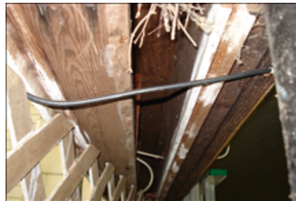
Underside of Addition, Uninsulated Gap
